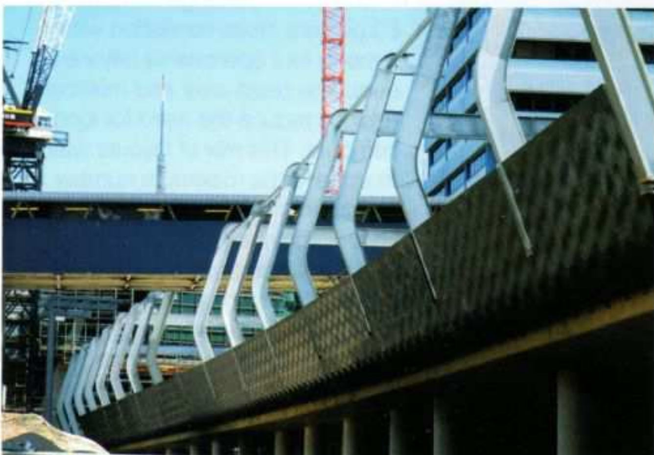
The 'ribs' (shaped like a whale's rib cage) are the support structure designed to hold high voltage cables, while also visually defining the rail corridor.
